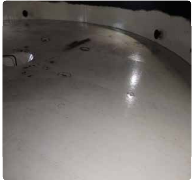
Tank bottom with an example of a marking with underside corrosion after completed tank bottom MFL-screening.
