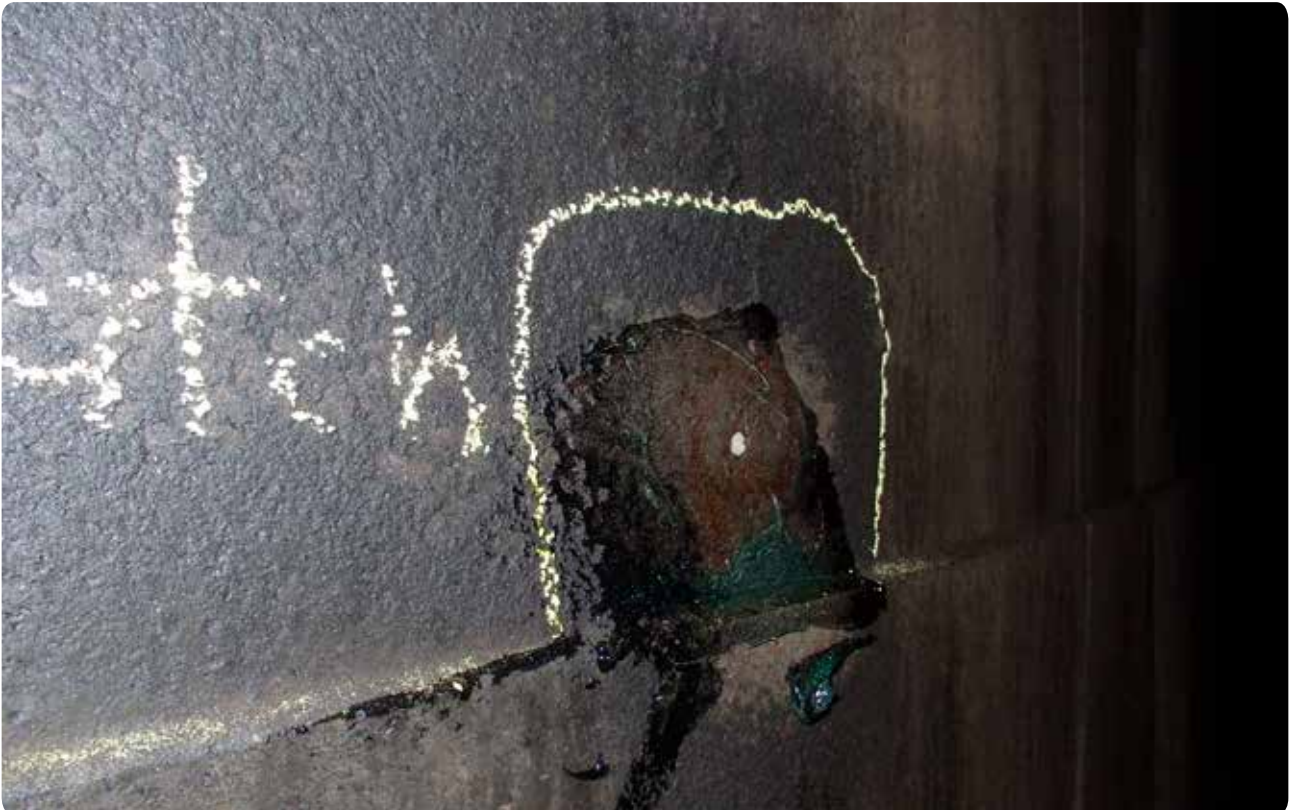
Through thickness corrosion on shell plate
