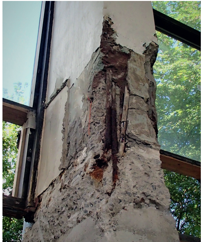
During the renovation of the existing concrete parts some corrosion was encountered and repaired.
